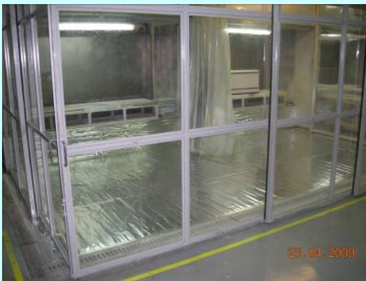
Paint booth enclosed by fixed panels
