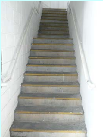
Staircase installed with anti-slip stair cover
